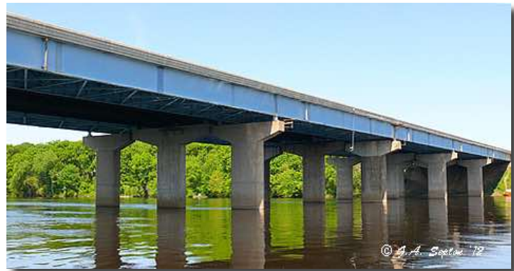
Above: The I90/94 Bridge as viewed from the east end looking west
